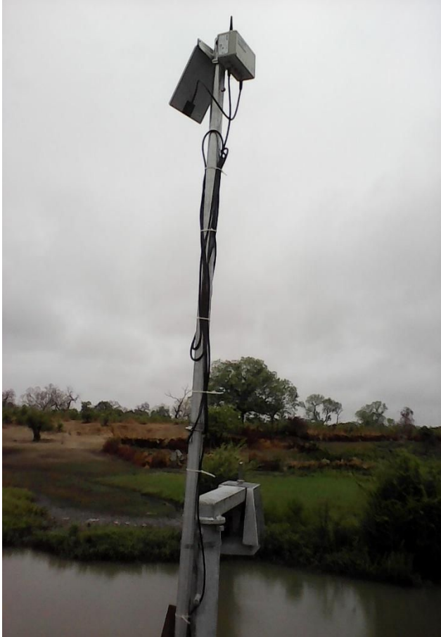
c) Image showing the infrastructure for the RLS and RLS and RTU at Sami Tenda
