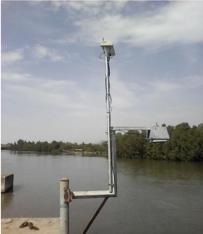
d) Image showing the installed RLS, RTU and solar Panel at Kerewan.
